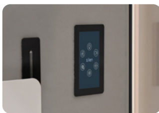
Air flow and lighting dimmer
